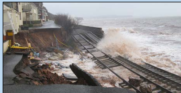
Damaged railway lines at Dawlish, 2014
